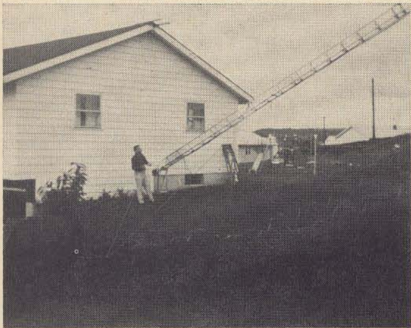
Tower on the way down with helpful neighbor demonstrating the use of the restraining lines.
